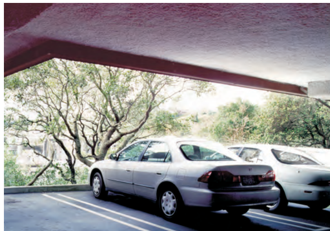
K-13 sprayed to this concrete parking deck provides thermal control to the conditioned spaces above.
